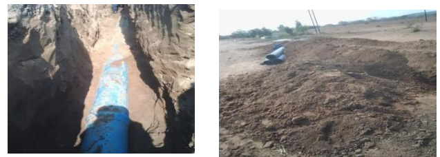
Figure 3. Raw water pipeline of the Moamba Village SSS Source: Authors.
